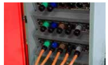
Emergency power systems
