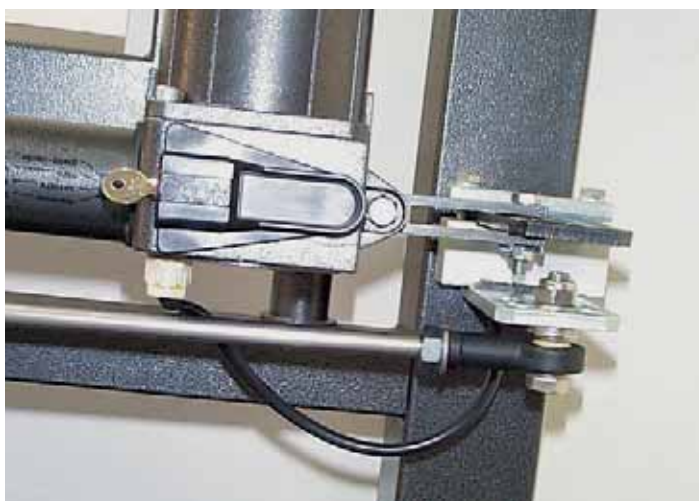
Picture 51.3: igubal® rod end bearings in the closing mechanism of an outdoor security gate
