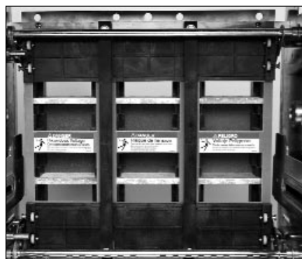
Figure 13 Safety Shutters in Open Position
