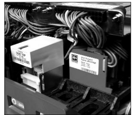
Figure 3 Shunt Trip Switch Installed
