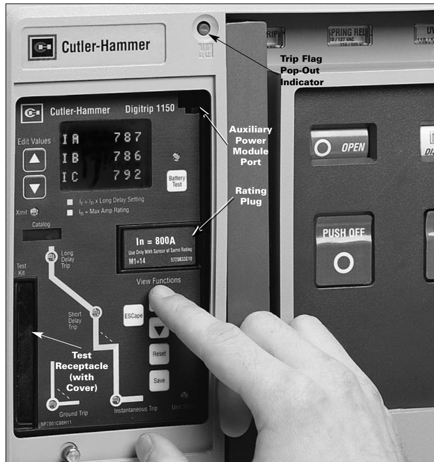
Digitrip RMS 1150 Programmable Trip Unit Installed
