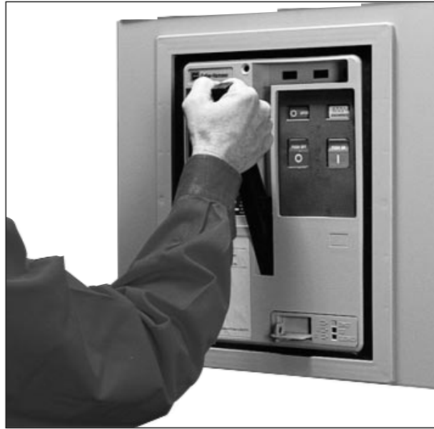
Magnum Circuit Breaker Being Manually Charged
