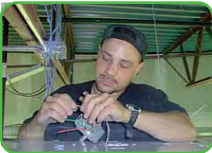
Push-wire connectors used in a cable duct with double power outlet.
